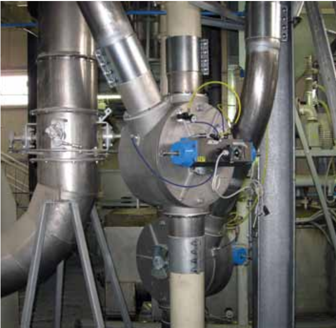
VAR Diverter Valves in pneumatic conveying system
