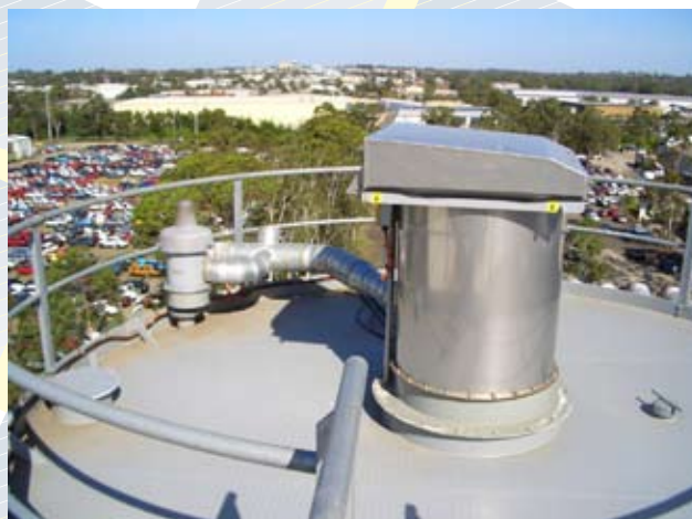
VHS Valve and SILOTOP® R01 in CONCRITE Concrete Plant in Sydney, Australia
